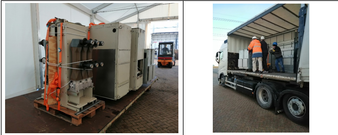
Figure 9 Transport activities for the electrical breaker cabinets to be donated by Germany and the Netherlands to the HEAF 2 Project; a) cabinets prepared for transport (left), b) cabinets being loaded on a truck (right)
