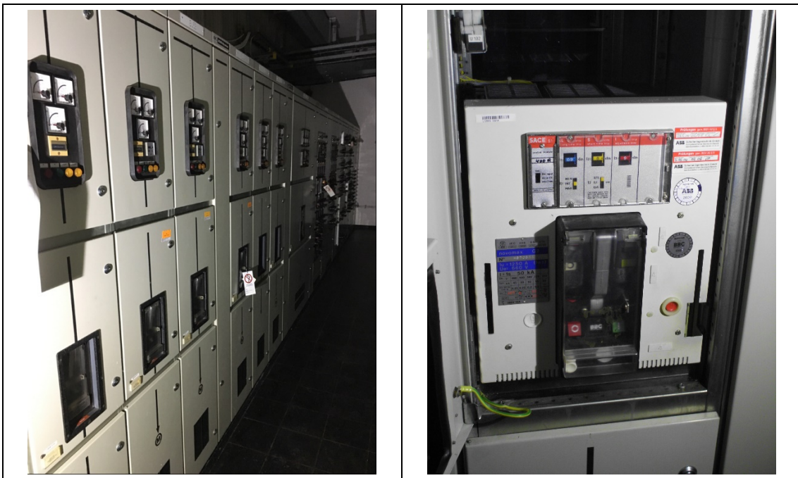
Figure 8 Medium voltage breaker cabinets; view from the outside (left), and breaker inside (right)
