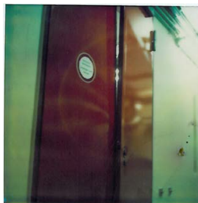
Figure 3 Fire door damaged according to a HEAF fire event; photograph from outside the fire compartment, from [2]
