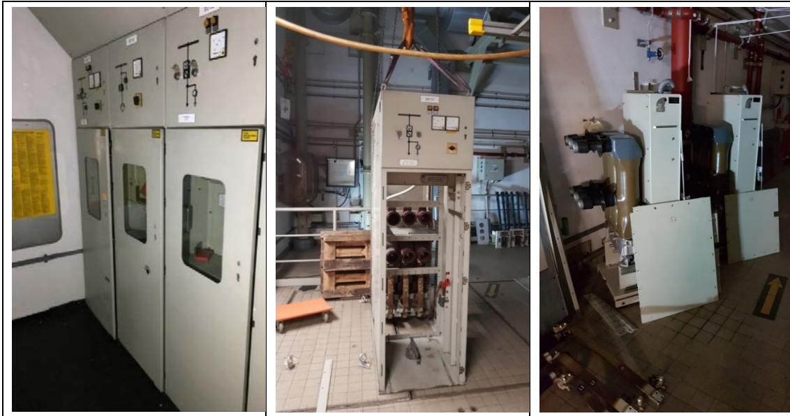
Figure 7 High voltage breaker cabinets; view from the outside (left), open cabinet enclosure (middle), and breaker itself (right)
