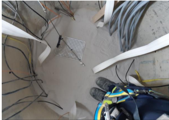
Fig. 3.52 Installation of ES3 in Shaft 1 with metal tube of back-up hydration system
