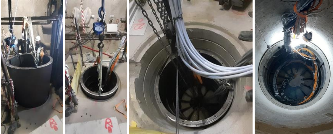
Fig. 3.59 Sequence of inserting the bottom section of the metal plug into Shaft 1
