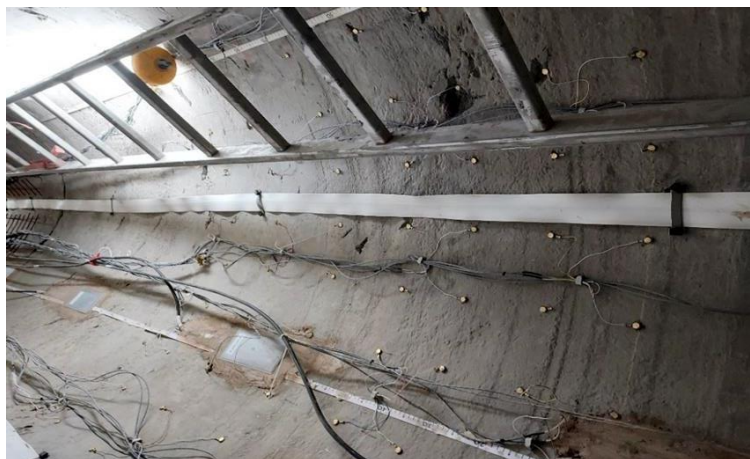
Fig. 3.81 Vertical TDR sensors installed at the wall of Shaft 2
