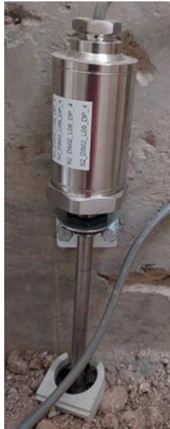
Fig. 3.68 Vertical displacement sensors in Shaft 2
