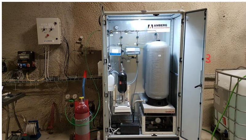
Fig. 3.62 Hydration system for Shaft 1
