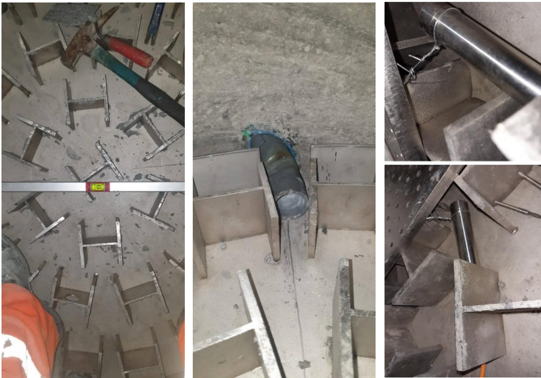
Fig. 3.43 Installation of the pressure chamber, the connection to the feeding borehole (middle) and the pressure chamber sensors (right) for Shaft 1
