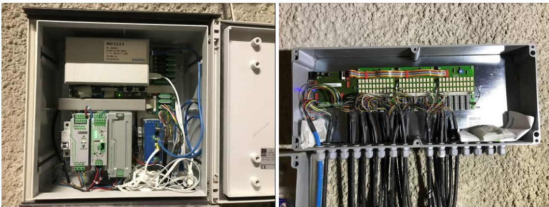
Fig. 3.95 Glötzl acquisition PC and multiplexer MUM30
