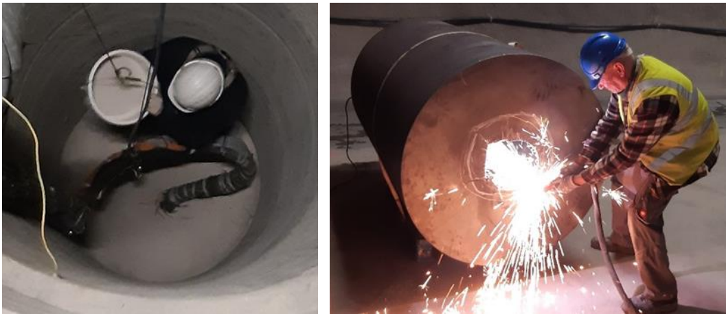
Fig. 3.58 Centering the cable harness within the additional sand layer (left) and widening of the hole in the lower confining tube (right) for Shaft 1
