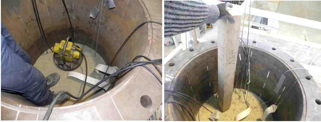
Fig. 5.40 Compaction of the DS using a vibratory plate in HTV-7 (left) and compaction of the DS using a square timber (right)
