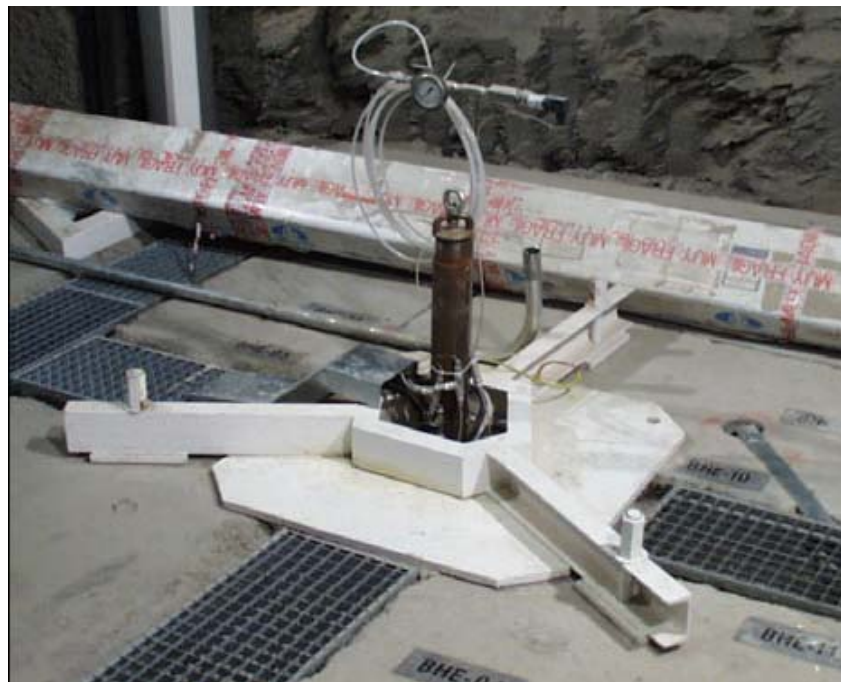
Figure 2-4 Heater borehole BHE-0 with the steel lid anchored to the rock
