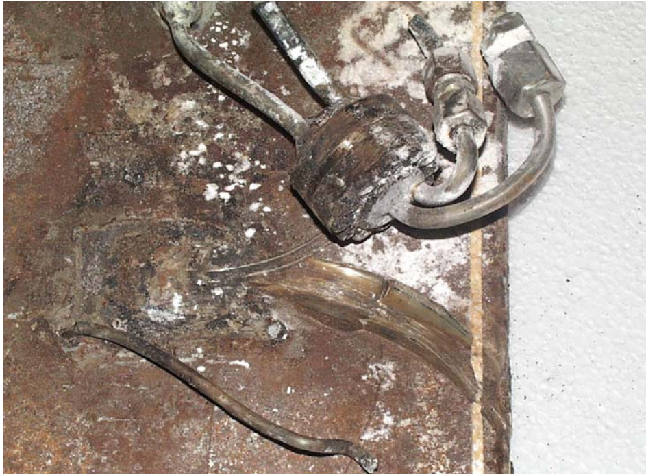
Fig. 5.4.5 Pressure gauge 61966 (upper side) – damaged by the continuous miner during drift excavation
