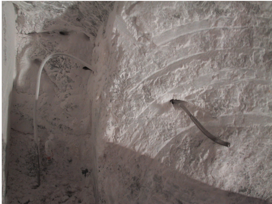
Fig. 5.2.1 Temperature gauge in situ with the PT 100 sensor at the drift wall and the measuring cable in the cable slot (cross section I1)
