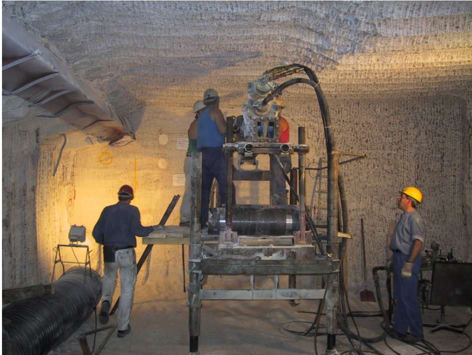
Fig. 3.7 Cored drilling in the excavated test drift. The drift was widened into the surrounding rock salt to enable the retrieval of the heater casks
