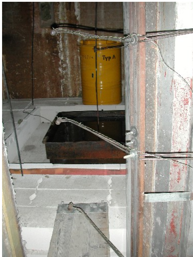
Fig. 2-8 View of the fire compartment through the front door
