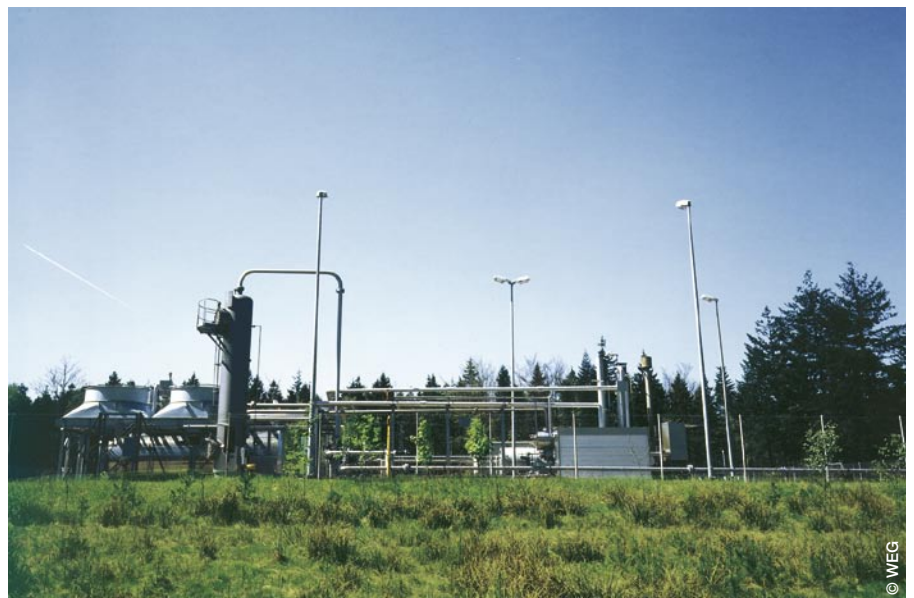
▲ Gastrocknungsanlage Gas dehydration facility
