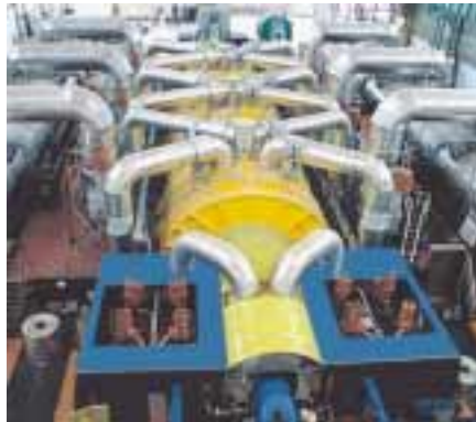
▲ 1000 MW-Turbogenerator 1000 MW turbine generator
