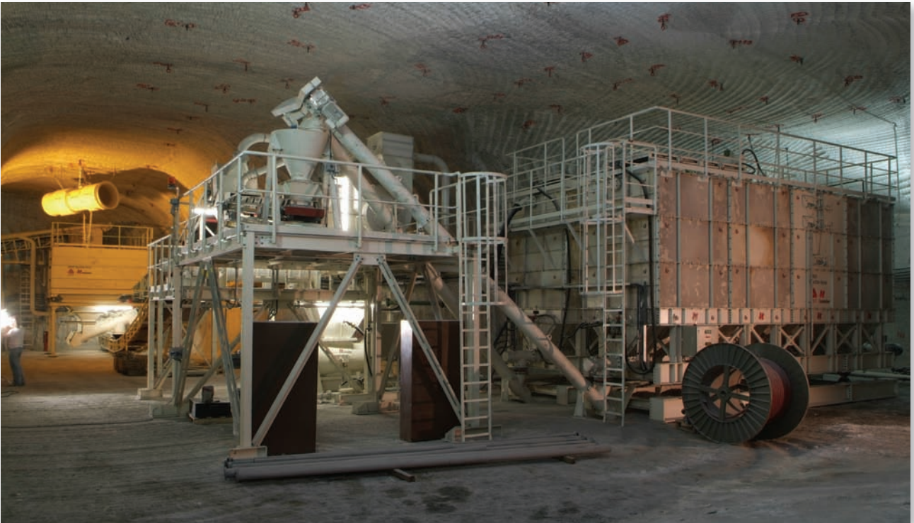
▲ Fig. 15: This photo shows where rock salt and bonding agent (MgO) are blended. The unit is on the 700-m-level.
