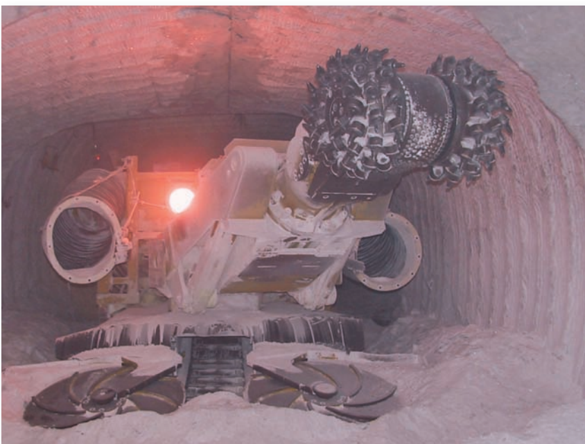
◀ Fig. 14: This photo shows a part-face heading machine ready to cut loosening in a gallery which is prepared for building a flow barrier.
