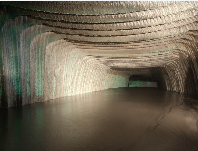
◀ Fig. 13: Sorel concrete is poured in the prepared gallery on this photo. The concrete extends very evenly.
