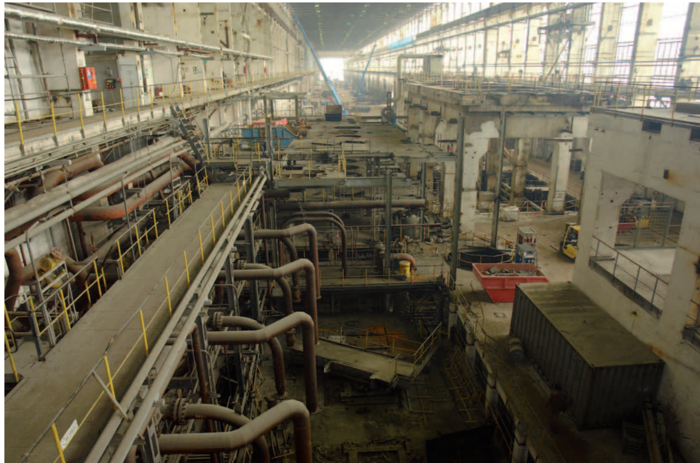
Fig. 41: Turbine building of the Greifswald nuclear power plant after removal of the generators
