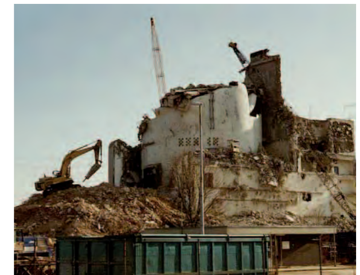
Fig. 17: Conventional demolition of the outer building shell of the Niederaichbach nuclear power plant
