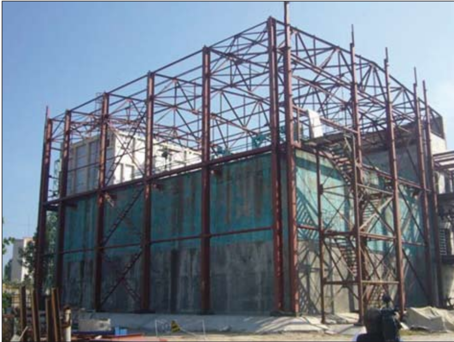
Fig. 5. Facility for retrieval of solid waste – ICSRМ – above the concrete bunker.
