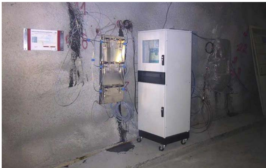
Figure 2-21 Measuring cabinet for monitoring pore-water pressure and temperature
