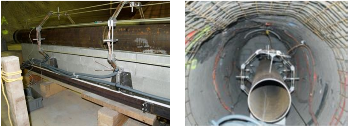
Fig. 4.3 HE-E experiment module (heater liner, bentonite blocks and buffer sensors) before (left) and after (right) installation in the microtunnel
