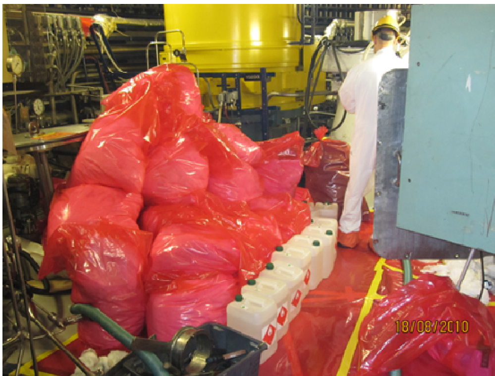
Figure 2 Unallowable fire load and flammable liquids during outage 2010 inside containment
