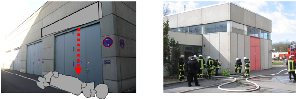
Figure 6 Blocked building entrances due to fallen concrete elements
