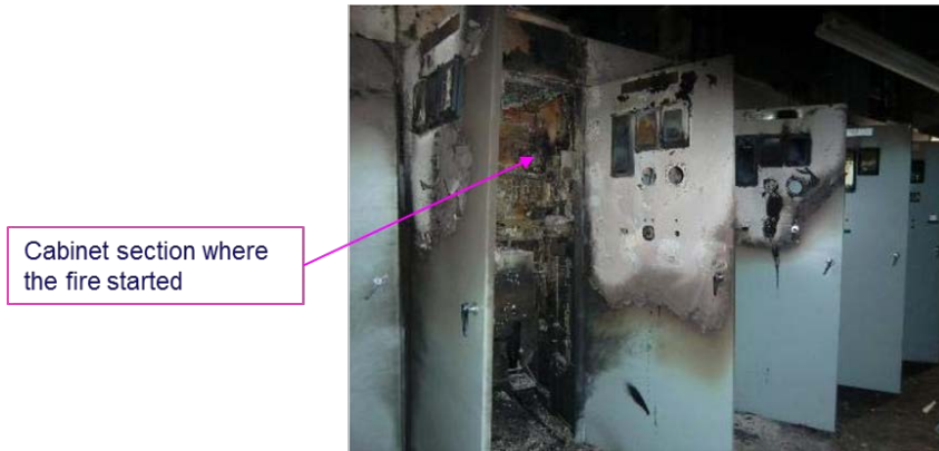
Figure 1 Electric cabinet with the sector where the fire started and others impaired [4] (Onagawa NPP in Japan on March 11, 2011)
