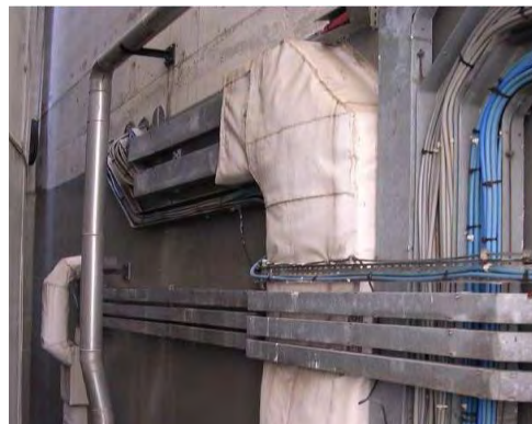
Figure 17 Cable tray wrapping installed outside after 25 years lifetime
