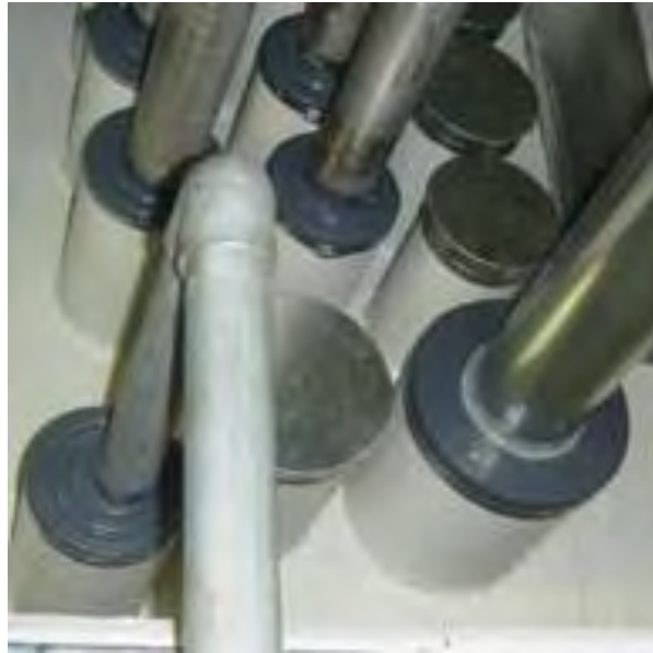
Figure 1 Pipe penetration seals of non-combustible pipes sealed by reversible silicone expansion joints and one reserve pipe seal closed with a sheet metal cap (bottom-middle and top-right); image source: G+H Isolierung GmbH, www.guh-brandschutz.de
