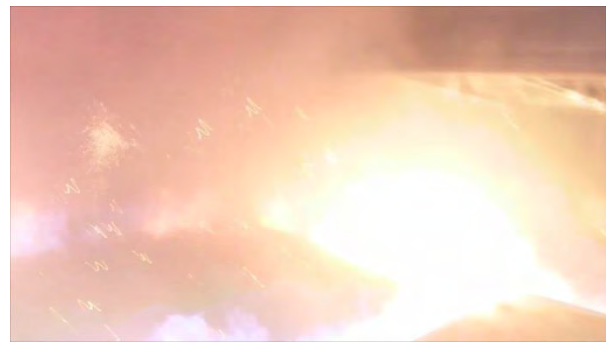
Figure 10 Low voltage HEAF; top of cabinet; cable tray visible in upper right of photo
