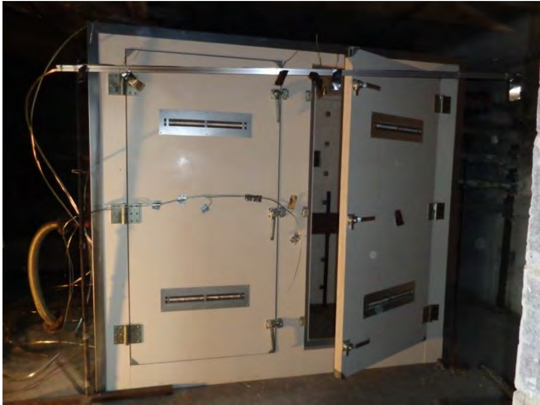
Figure 14 Casing around electrical cabinet as potential fire source
