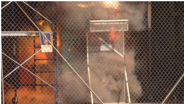
Figure 9 Low voltage HEAF; front of cabinet
